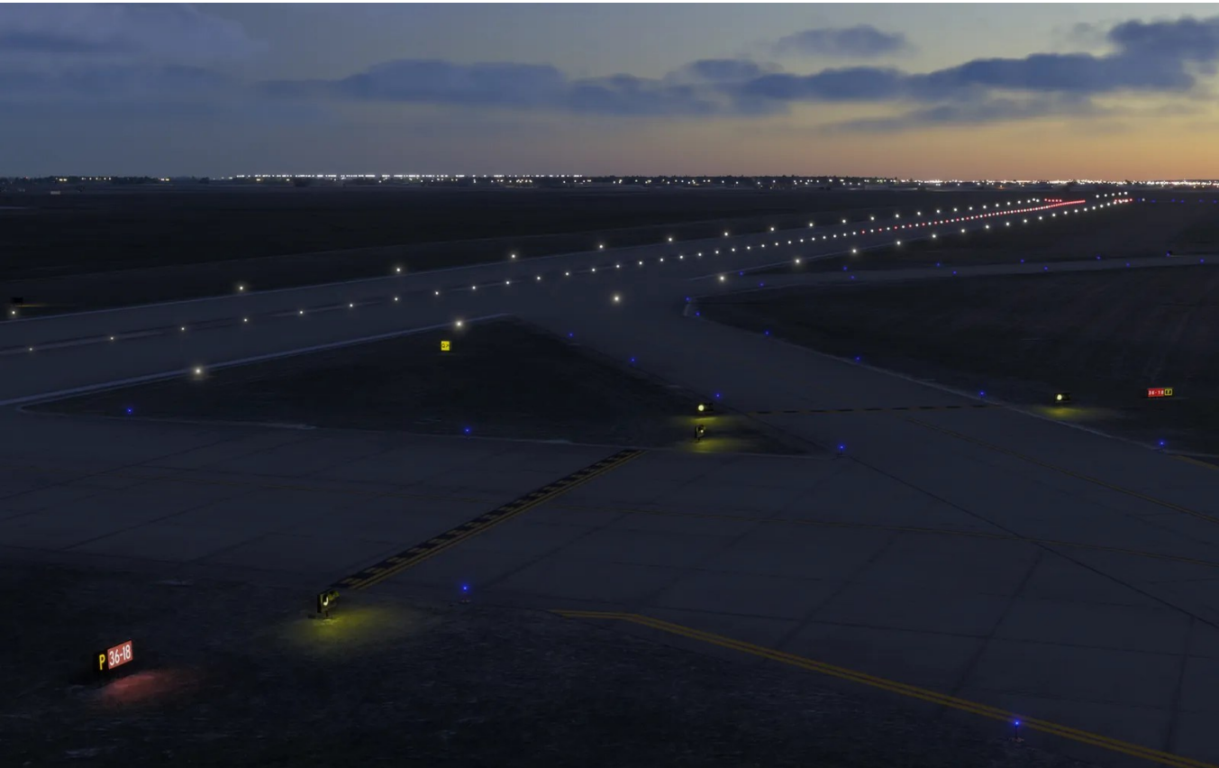
Taxiway and runway lighting at dusk
